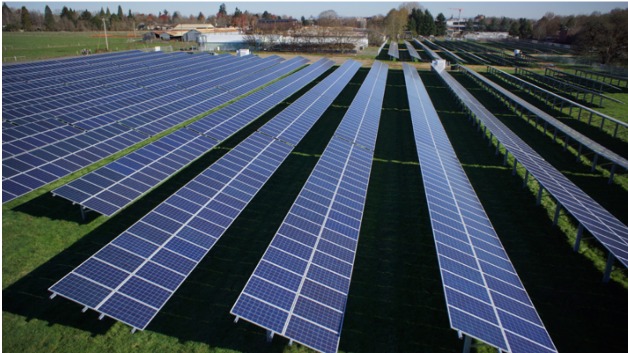
1.435 megawatt 35 th Street solar array
